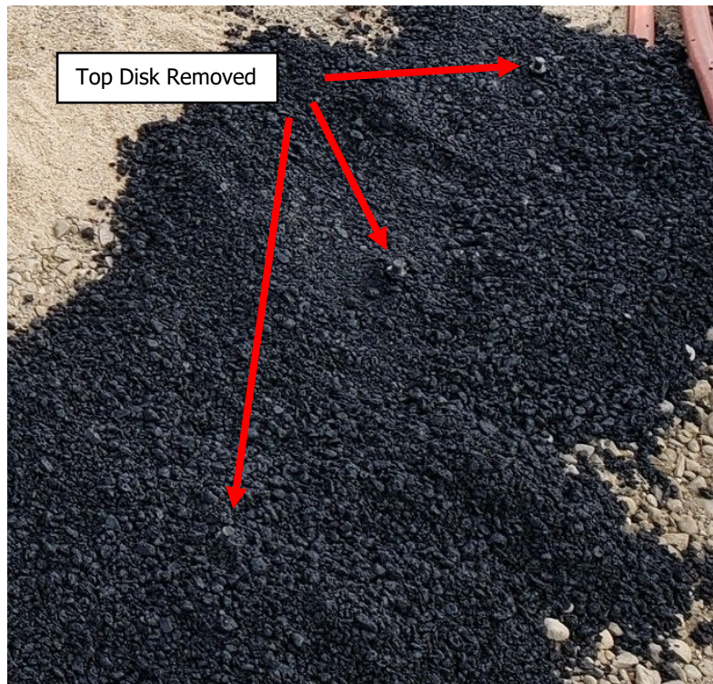
Figure 11: Exposed gage threads sticking above the asphalt.
