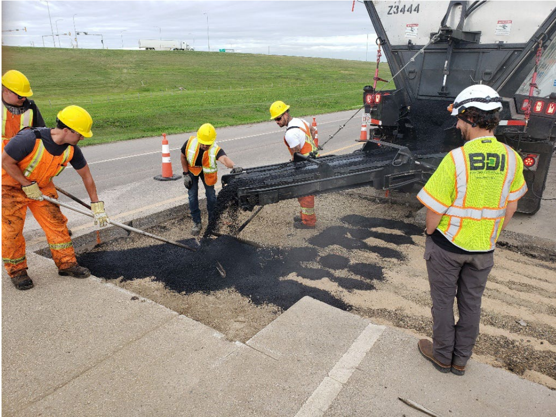
Figure 7: Cover with asphalt as in normal paving operation. Then compact to the desired compaction for the paving operation.
