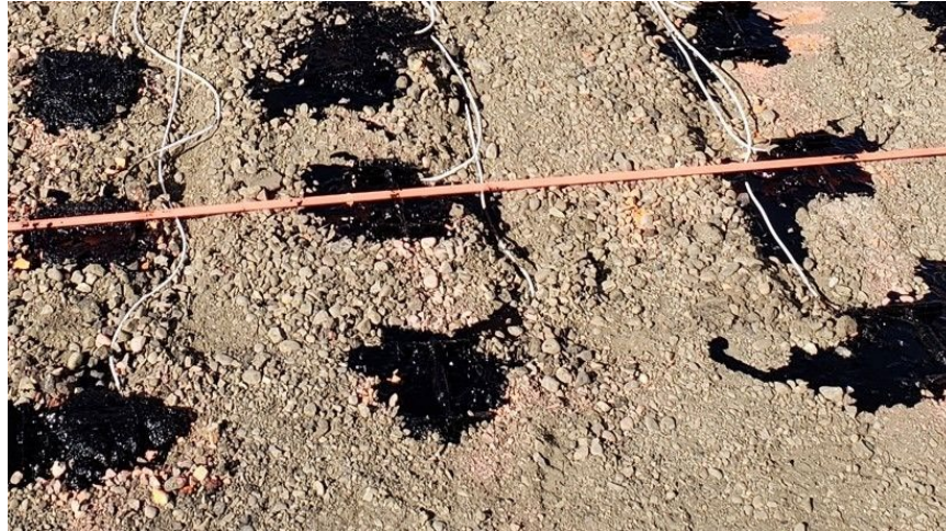
Figure 4: Sensors are covered with a thin layer of asphalt primer to the leveled base or subgrade surface at each location. The primer should completely cover an area 6 in x 10 in sq.
