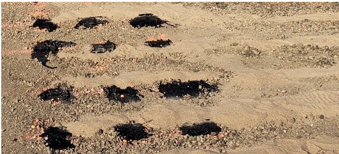
Figure 5: Lead wires will be routed from each sensor in a 2-in deep slit trench leading to the shoulder edge.
