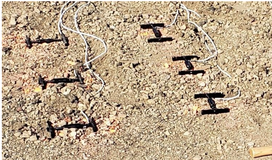
Figure 3: AST350-6, 6-inch Asphalt Strain Transducer laid out on top of the base course. Sensors are arranged in perpendicular orientation as shown. Be sure to record the serial number and location of each AST350 strain gage.
