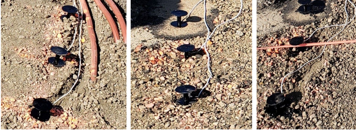
Figure 8: Be sure the gage has flat ground to stand on with the spike end embedded in the base course. Fill in around the base of the gage with mastic to hold the sensor in the vertical position. Fill wire trenches with sand for protection.
