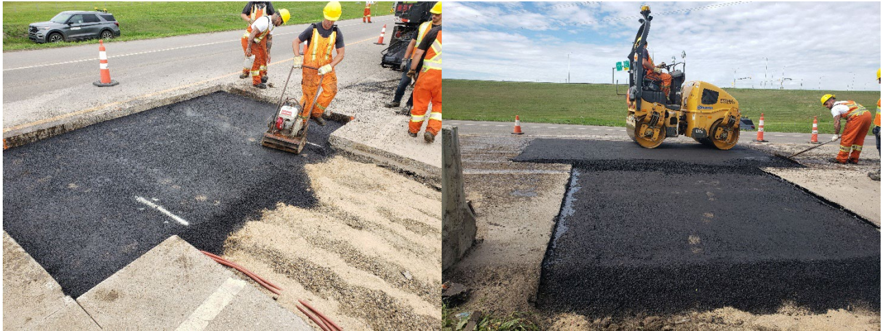
Figure 14: Continue the paving operation per usual. Start with the use of a gas-powered push tamper on the first few layers until a good amount of cover. Complete the paving using a conventional rolling compactor.
