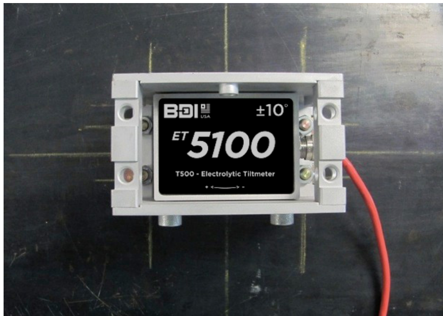
Figure 11: Tiltmeter Installed on Structural Member
